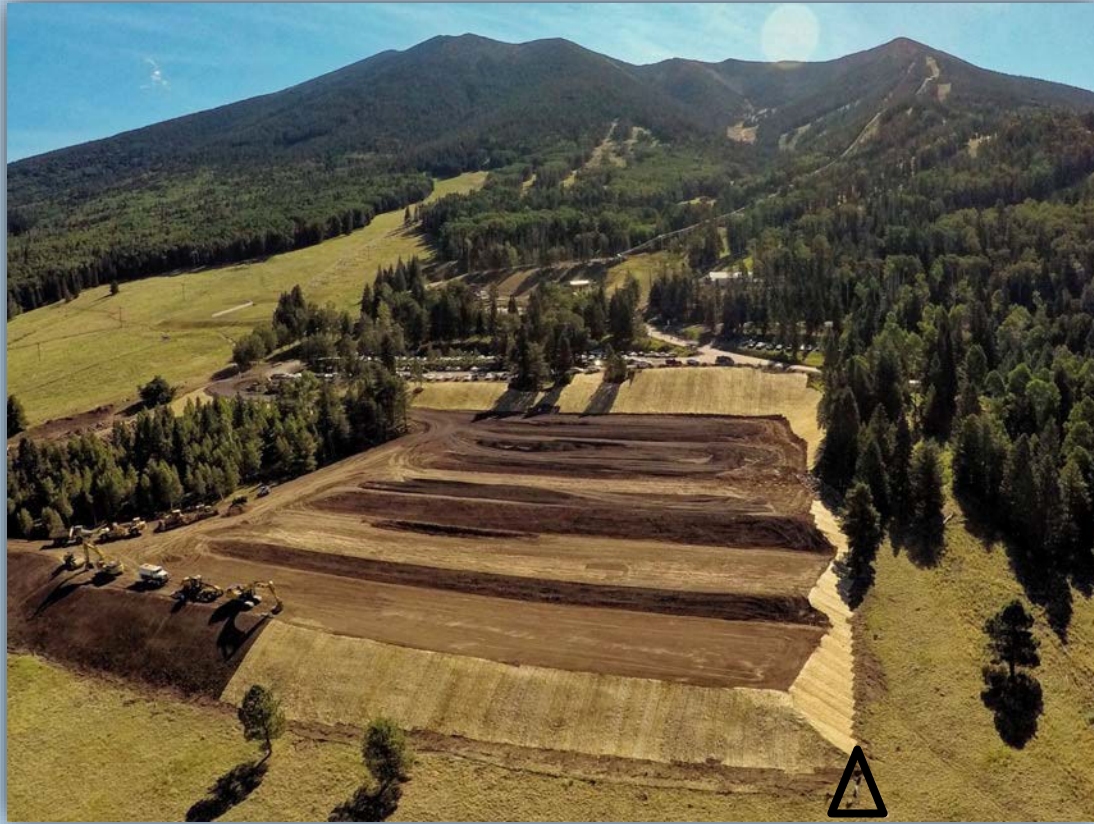
Arizona Snow Bowl's new parking lot under construction on Hart Prairie, summer 2020. Realignment of stormwater drainage system has exacerbated existing runoff problems on the prairie. Triangle is cadastral corner monument marking southwestern boundary of Arizona Snow Bowl's Special Permit Use Area.
